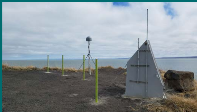
Stebbins/St. Michaels GNSS-R Station, AOOS/UNAVCO (photo courtesy UNAVCO)
